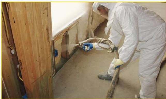
Equipment on the job: The crew used a Graco E-20 and Fusion AP spray gun to get the foam applied in all the cracks and crevices.
